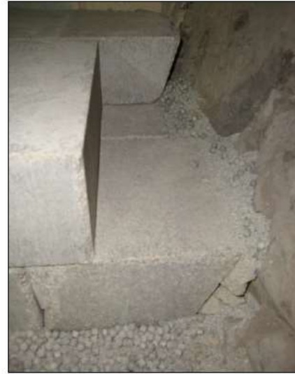
Figure 8 Installation of bentonite core, wall made with bricks, pellets/powder mixture between claystone and bentonite bricks. Background: hydration membrane
